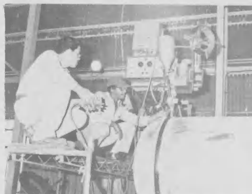
M. Werleman and E. Rumnit, welding the head of a bundle shell with an automatic submerged welding machine.
